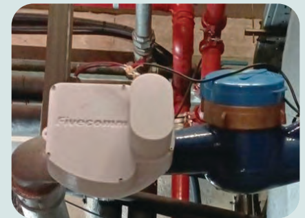
Figure 3. The 5G-LITE device (left) connected to a water meter (right) in a trial.
