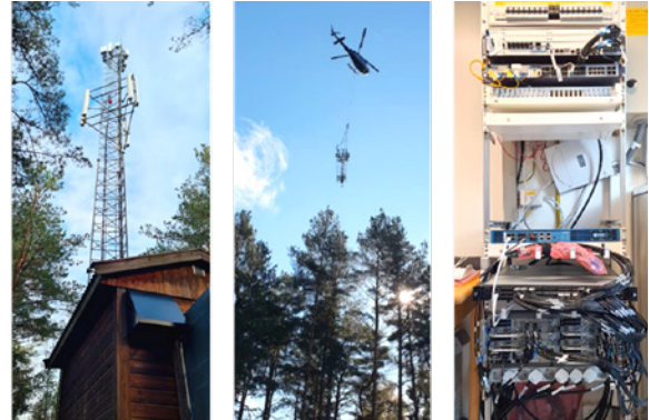
Figure 3: Picture of the Huawei gNB (3.6GHz and 26GHz) and eNBs (2.1 GHz) in the military location. Extended mast installed by 5G-VINNI. Edge Cloud (right)
