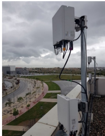
Figure 2: 5G deployment at Ada Byron building
