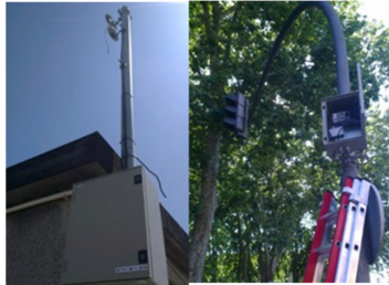
Figure 30: RSUs mounted in the municipality building and in a traffic light
