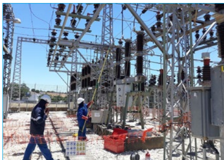
Fig. 70: Garraf Natural Park Primary substation
